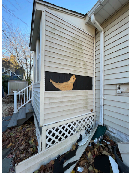
east addition (note no foundation, plywood and vinyl only)
