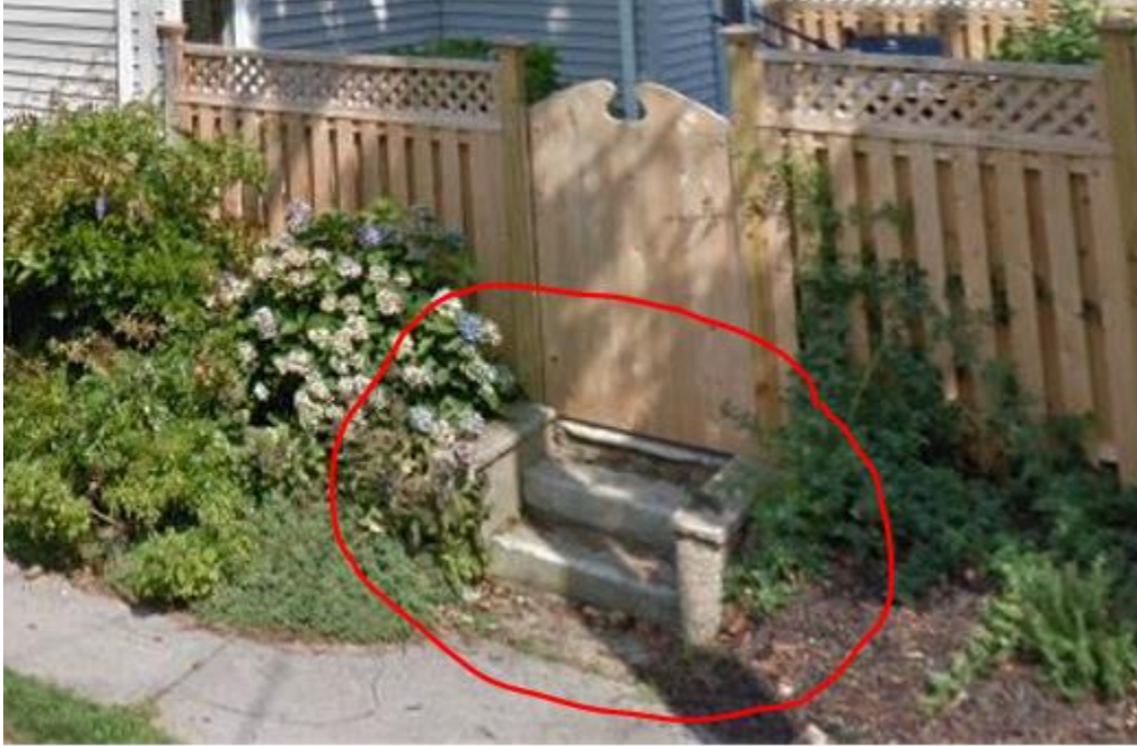
Photo notes: Existing concrete landscape stair on New York Avenue, which provides access to the rear yard, which is located approximately 2' higher than the existing sidewalk grade elevation.
