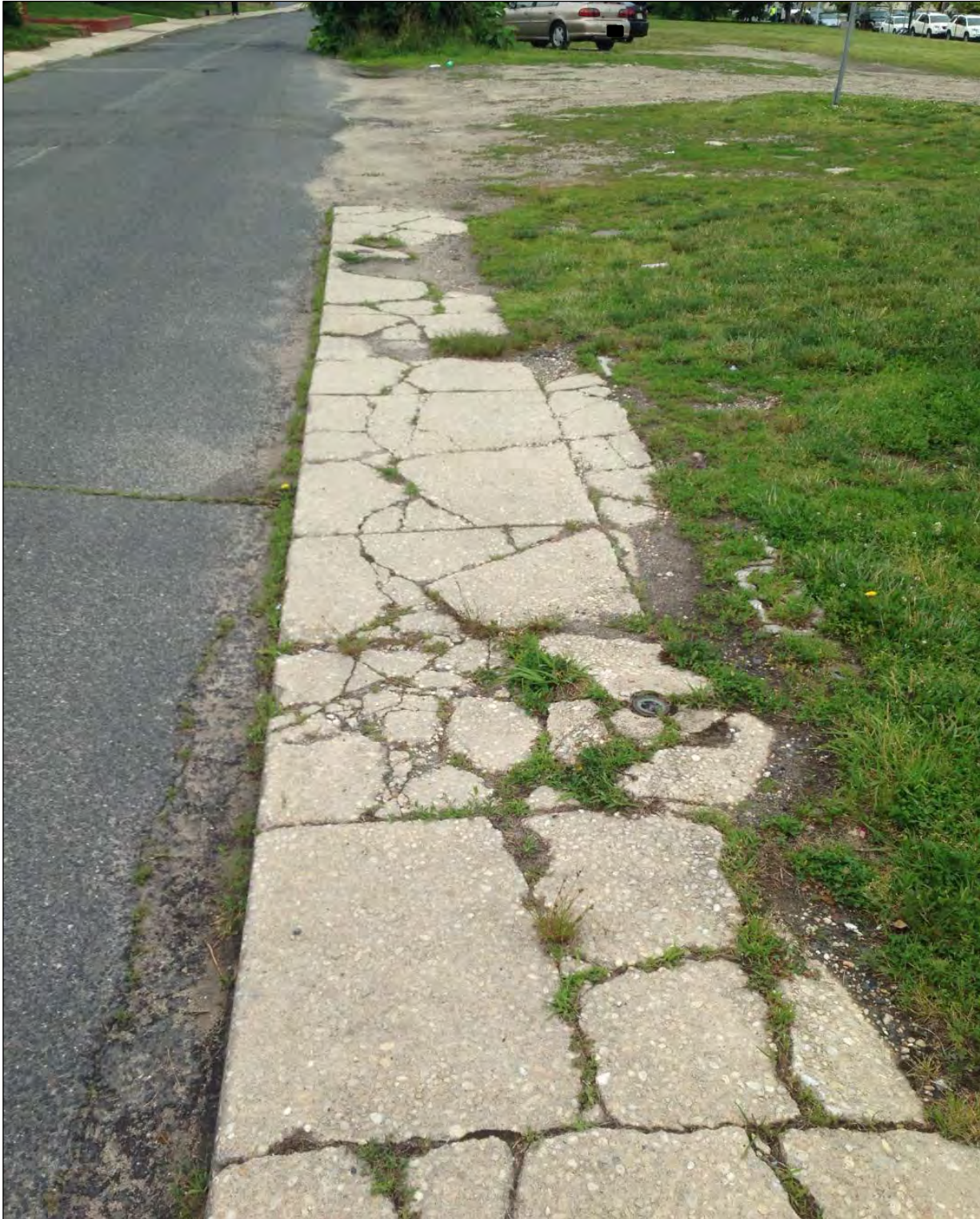
Damaged sidewalk on Lot 39.01
