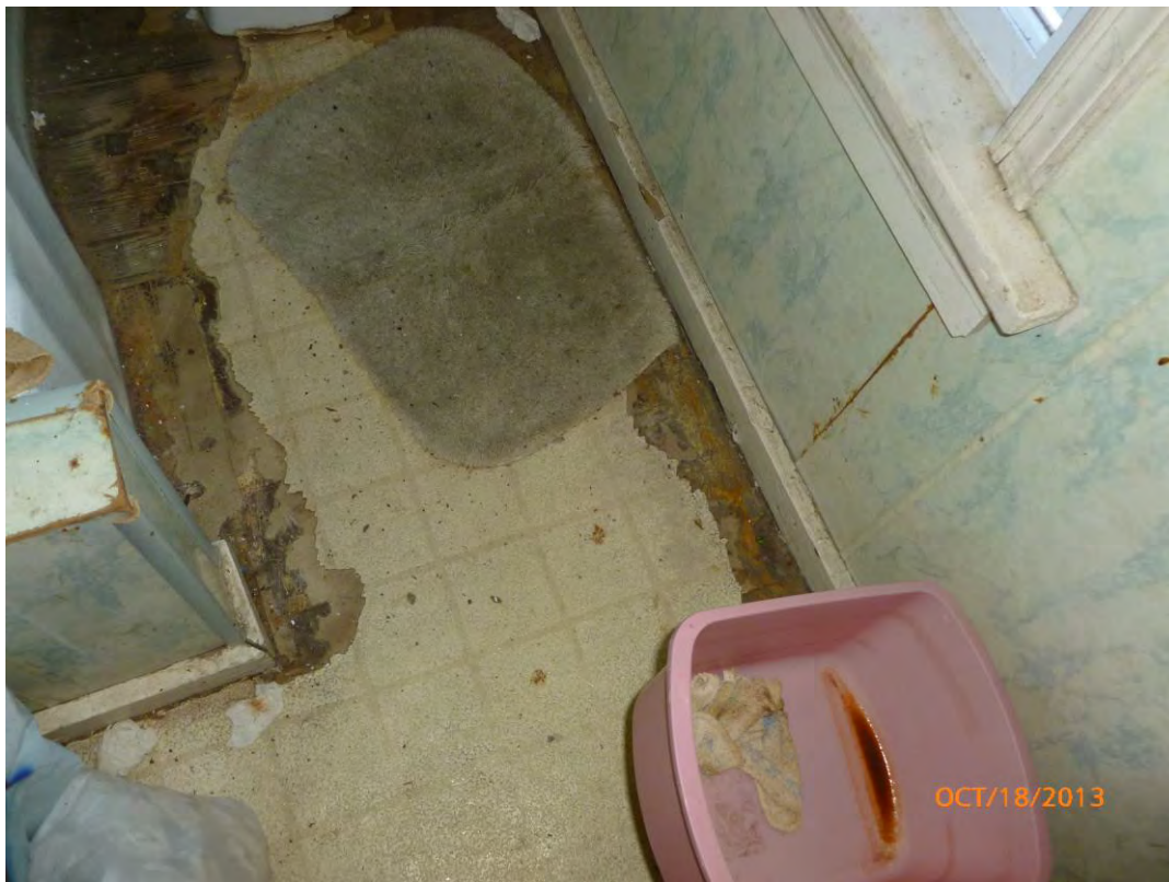
Photo 5 - 1 ST Floor, Kitchen: Beige linoleum with other layers underneath ( note : mid-layer identified to be ACM and, therefore, all layers must be treated and removed as asbestos).
