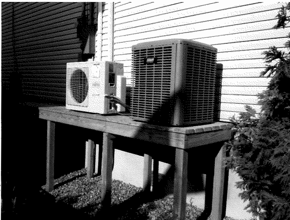
A/C PLATFORM 21 ALBANY ROAD NEPTUNE, NJ AUGUST 5, 2014
