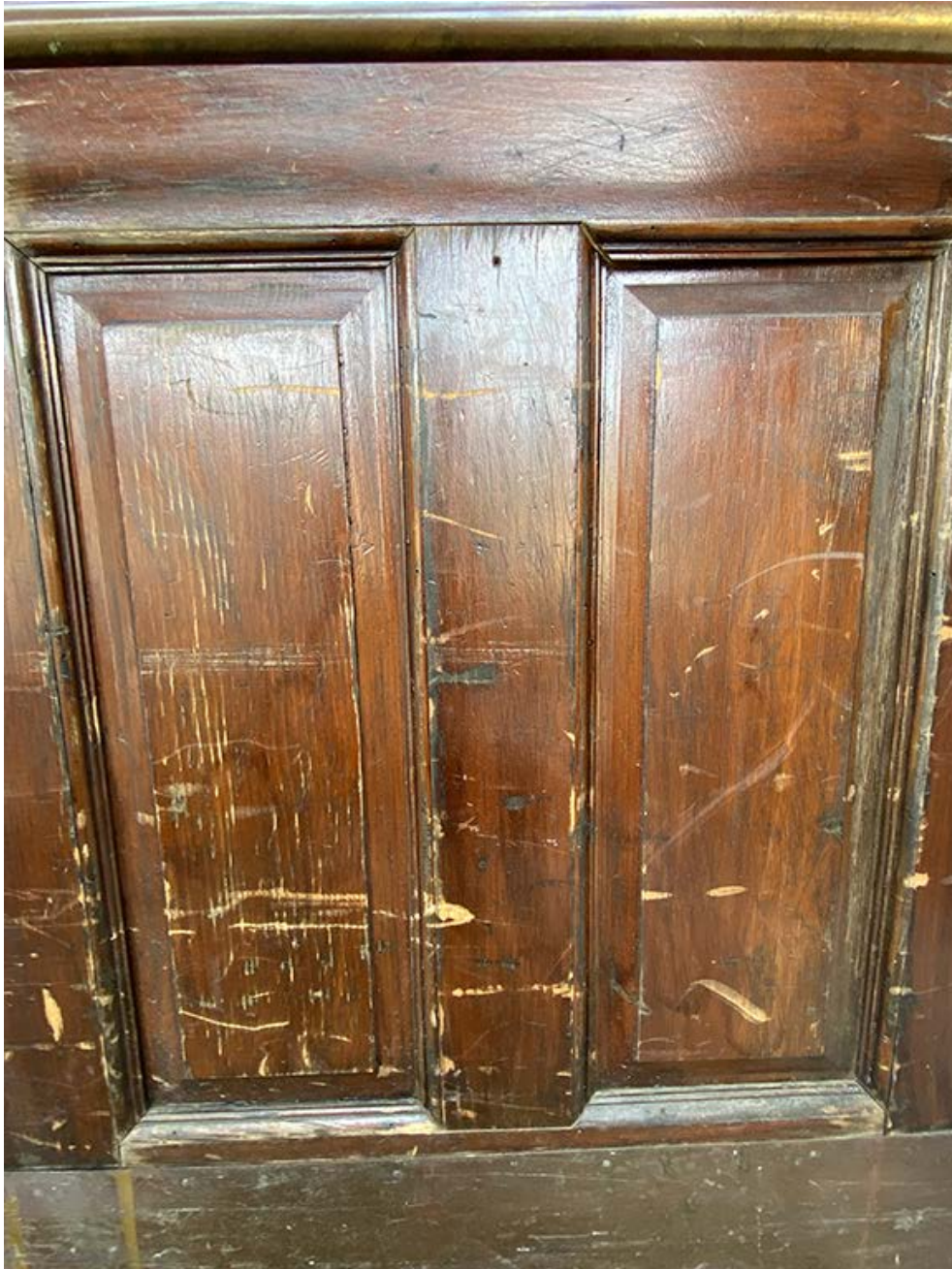
Inside door is not painted
